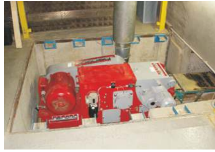
RHZ 400 S set up below ground
